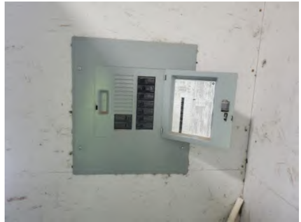
0042091e 4/2/2024 Main distribution panelboard for Hay Barn Hay Barn
