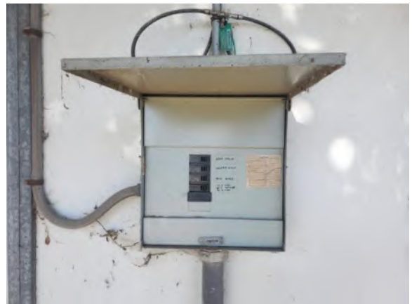
0042063e 4/2/2024 Main distribution panelboard for Barn Barn 1-29, exterior
