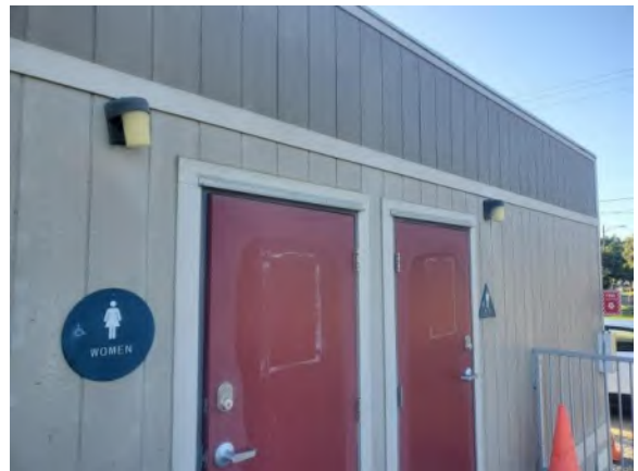
0042003e 4/2/2024 Surface-mounted, single lamp exterior lighting Restroom Building, exterior
