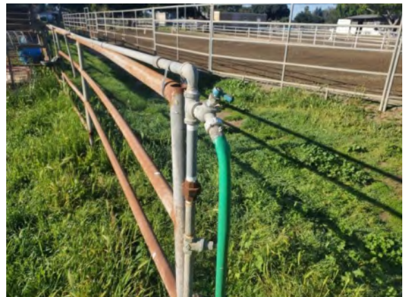
0042030e 4/2/2024 Galvanized steel pipe and hose bib Stalls 152-158
