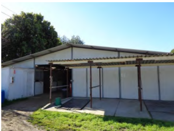
0042039a 4/2/2024 Composite metal clad wall panels, open to breezeway, and corrugated metal roof over grooming area Barn 1-29, north elevation
