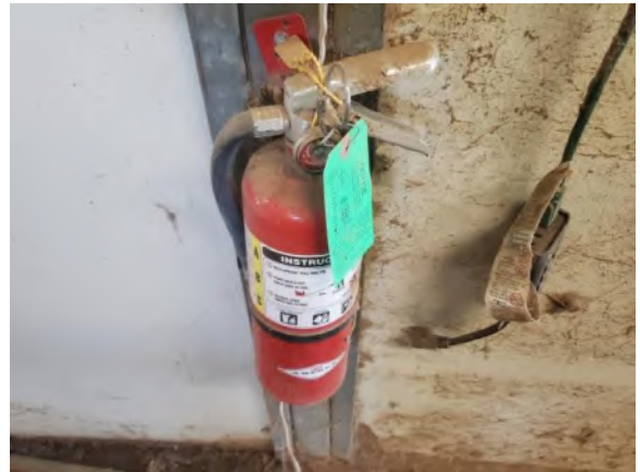
0042056e 4/2/2024 Fire extinguisher Barn 1-29
