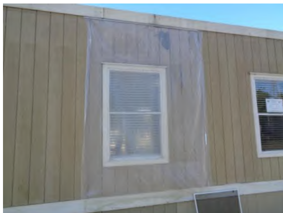
0042012a 4/2/2024 Deteriorating plywood siding and plastic sheeting over leak Office, north elevation
