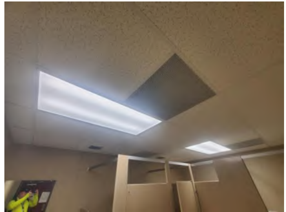
0042004e 4/2/2024 Recessed interior light with fluorescent lamps Restroom Building, men's restroom
