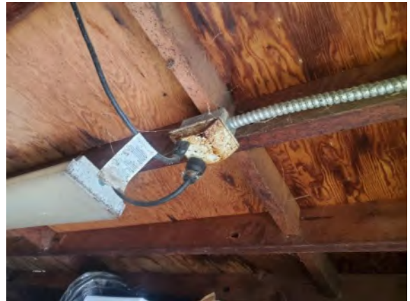
0042080e 4/2/2024 Interior electrical outlet Wood Tack Shed 7-8
