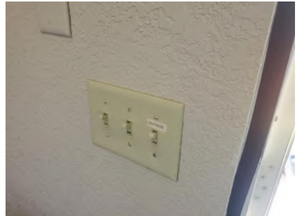
0042017e 4/2/2024 Light switches Office, lobby
