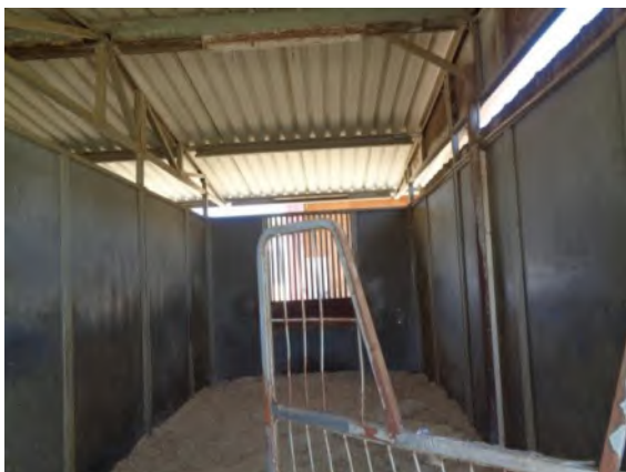
0042051a 4/2/2024 Typical stall with metal clad composite wall panels Barn 30-39, stall interior
