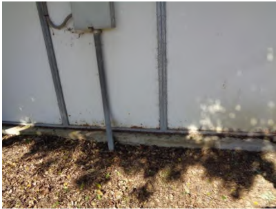
0042043a 4/2/2024 Minor rusting of composite metal clad wall panel frame Barn 1-29, east elevation
