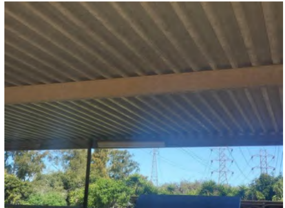
0042082e 4/2/2024 Surface-mounted lighting Stalls 81-89
