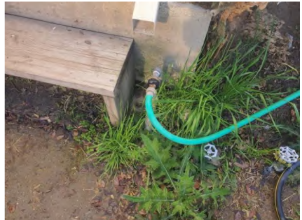
0042029e 4/2/2024 Galvanized steel hose bib Wash Rack 1, exterior
