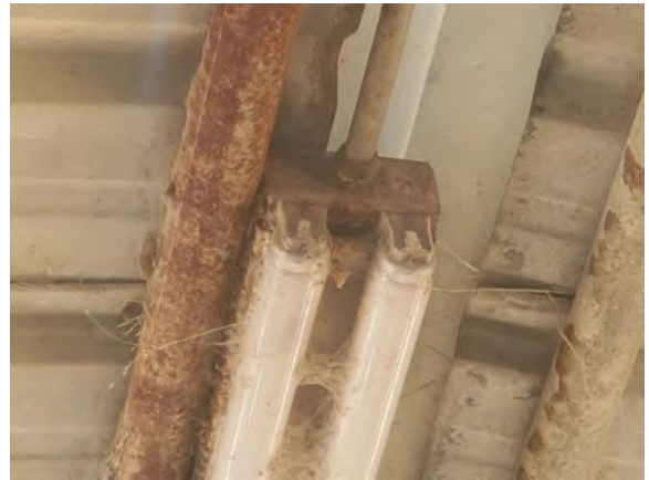
0042076e 4/2/2024 Corroded light fixture Stalls 47-62
