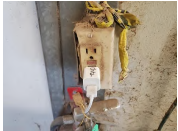
0042055e 4/2/2024 Damaged GFCI electrical outlet Barn 1-29
