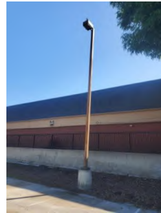
0042064e 4/2/2024 Pole-mounted road and parking light Site along entrance drive
