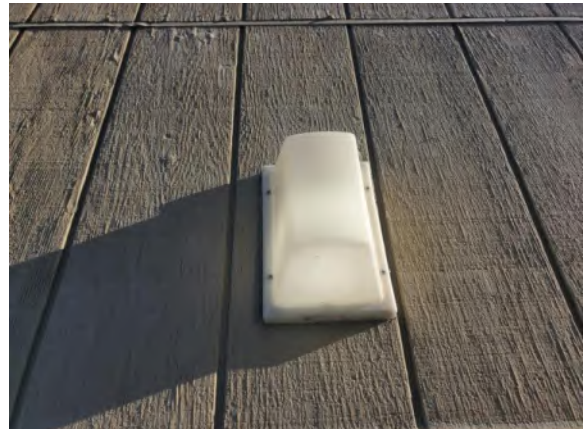
0042023e 4/2/2024 Surface-mounted, single lamp exterior fixture Office, exterior
