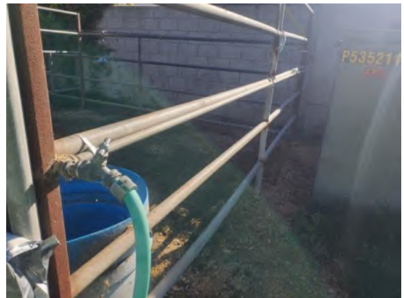
0042045e 4/2/2024 Galvanized steel pipe and hose bib Stalls 173-180
