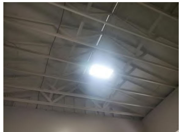
0042087e 4/2/2024 Surface-mounted interior lighting Hay Barn
