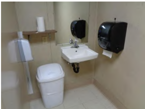
0042015a 4/2/2024 Wall-hung lavatory Restroom Building, women's restroom
