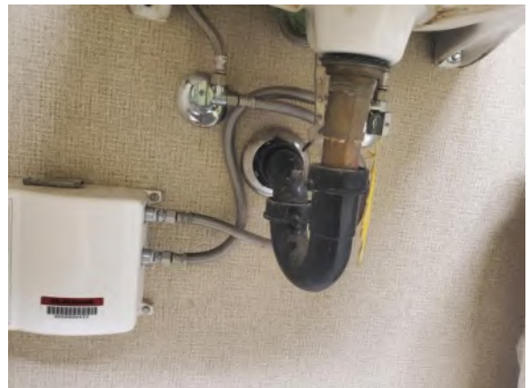
0042006e 4/2/2024 PVC waste piping Restroom Building, men's restroom
