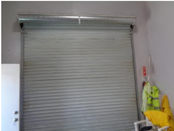
0042059a 4/2/2024 Manually operated overhead door Hay barn
