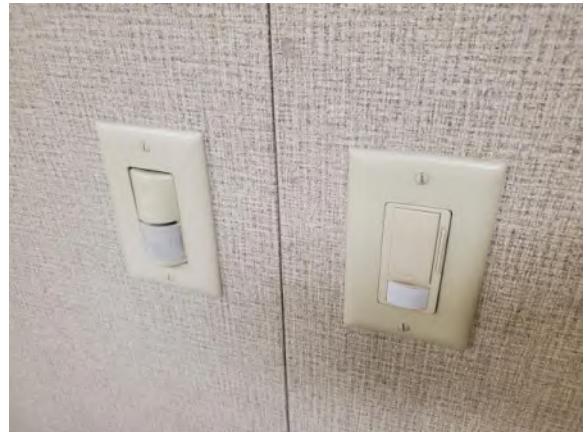
0042010e 4/2/2024 Light switch with integrated occupancy sensor Restroom Building, men's restroom
