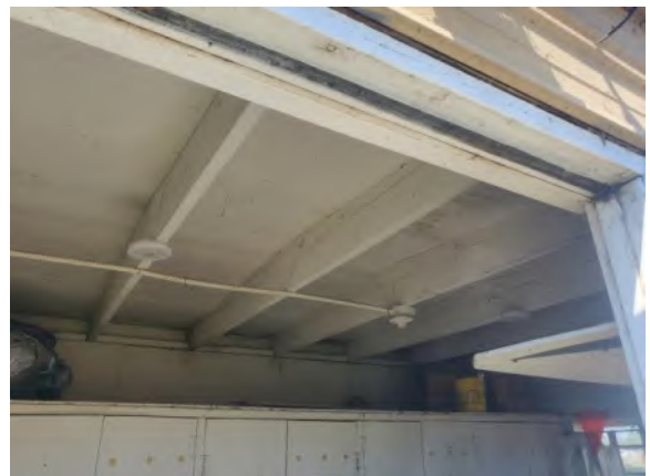
0042084e 4/2/2024 Lighting and electrical not in service Tack Shed 21
