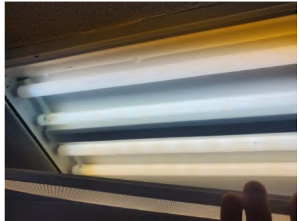
0042019e 4/2/2024 Fluorescent T12 lamps Office, lobby
