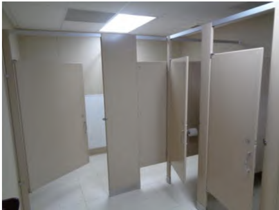
0042014a 4/2/2024 Suspended grid ceiling, FRP wall panels, vinyl tile floor, and painted metal partitions Restroom Building, women's restroom
