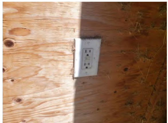
0042090e 4/2/2024 GFCI electrical outlet Hay Barn
