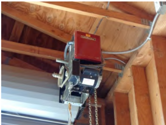
0042066a 4/2/2024 Electric opener for overhead door Hay barn
