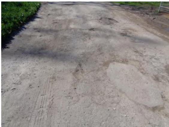
0042127a 4/2/2024 Potholes and patching Roadway
