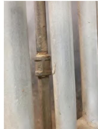
0042058e 4/2/2024 Galvanized steel water pipe Barn 1-29
