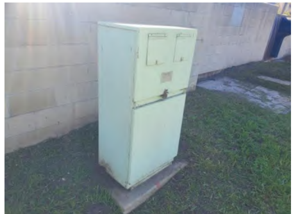
0042047e 4/2/2024 Utility-owned meter pedestal Site
