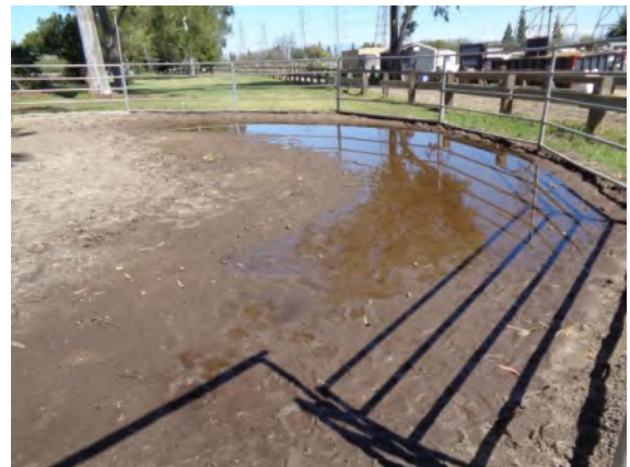
0042134a 4/2/2024 Standing water Turnout 8
