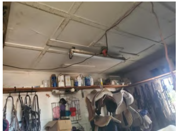
0042042e 4/2/2024 Surface-mounted lighting with T12 lamps Tack Shed
