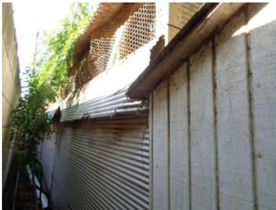
0042107a 4/2/2024 Corrugated metal siding on rear wall Stalls 170-172
