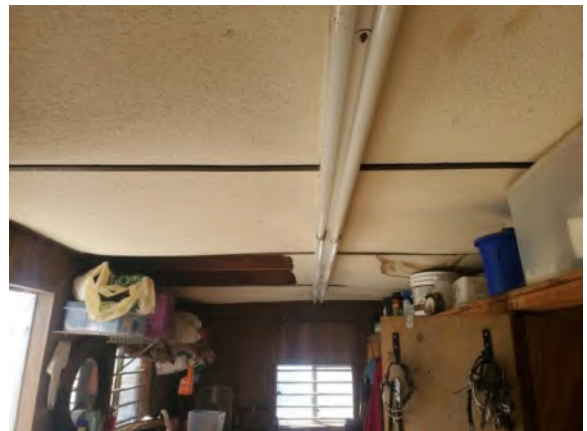
0042072e 4/2/2024 Surface-mounted lighting with T12 lamps Tack Sheds 9A, 9B, and 10
