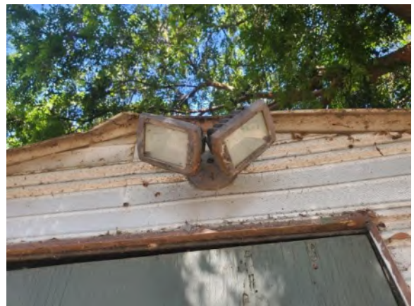
0042051e 4/2/2024 Surface-mounted HID light Shed, exterior
