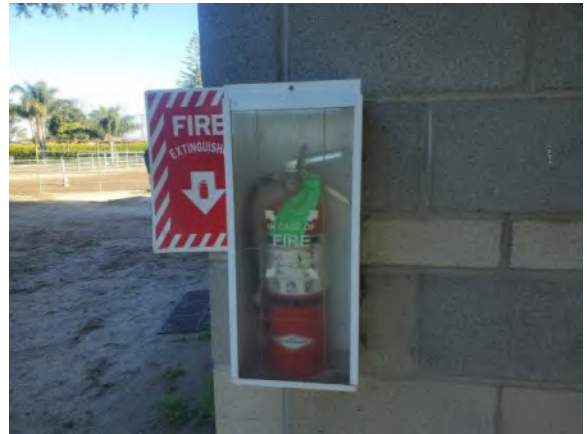
0042028e 4/2/2024 Fire extinguisher Wash Rack 1, exterior
