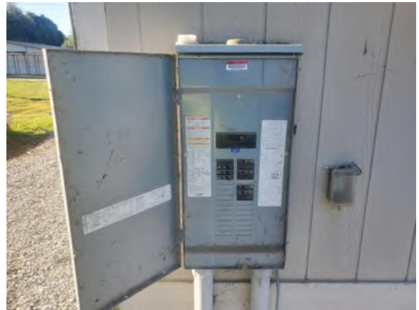
0042013e 4/2/2024 200-amp main distribution panel Restroom Building, exterior
