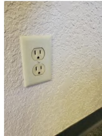
0042016e 4/2/2024 Typical electrical outlet Office, lobby
