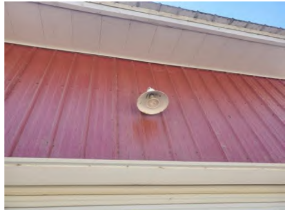
0042089e 4/2/2024 Sconce style exterior lighting Hay Barn
