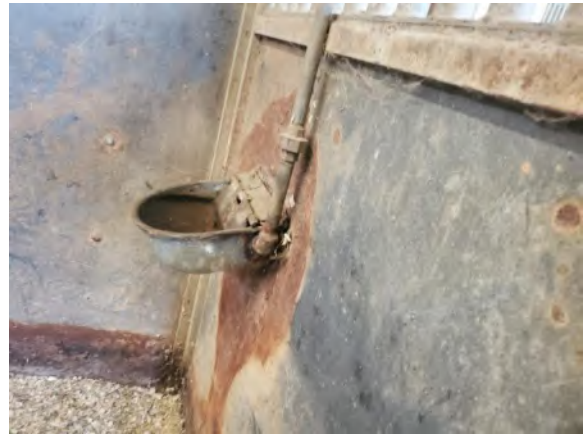
0042052e 4/2/2024 Corroded steel waterer Barn 1-29
