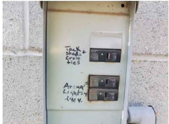
0042026e 4/2/2024 60-amp panelboard Wash Rack 1, exterior
