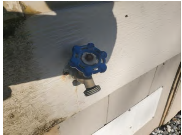
0042001e 4/2/2024 Exterior potable water hose bib Restroom Building, exterior
