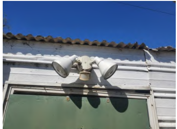
0042071e 4/2/2024 Exterior lighting Tack Sheds 9A, 9B, and 10
