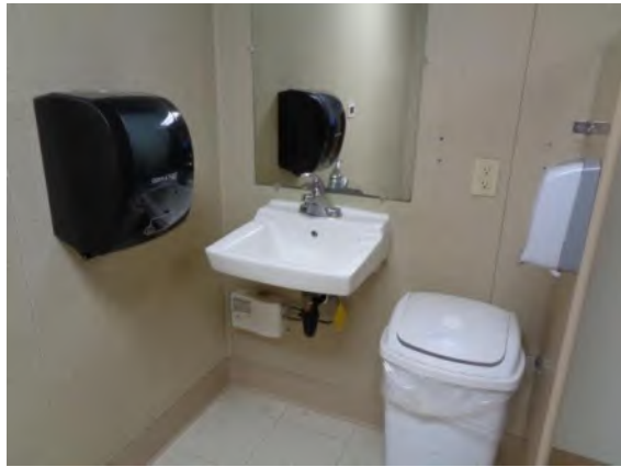
0042019a 4/2/2024 Wall-hung lavatory Restroom Building, men's restroom
