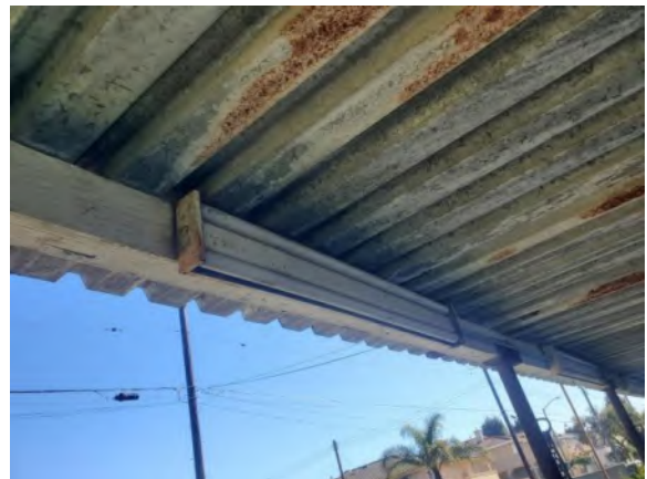
0042060e 4/2/2024 Slightly corroded surface light fixture with T12 lamps Barn 1-29, exterior
