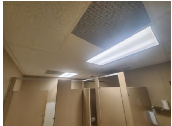
0042011e 4/2/2024 Overview of restroom systems Restroom Building, women's restroom
