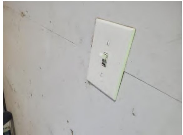
0042088e 4/2/2024 Typical light switch Hay Barn
