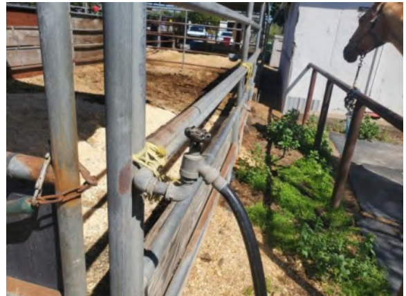
0042078e 4/2/2024 Galvanized steel pipe and hose bib Stalls 71-80
