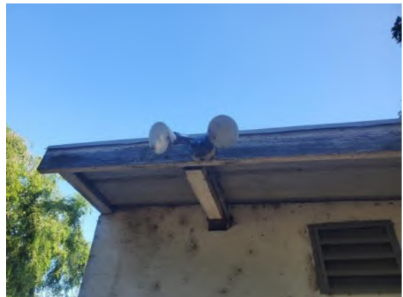
0042027e 4/2/2024 Exterior flood lighting Wash Rack 1, exterior
