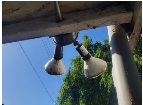
0042043e 4/2/2024 Exterior flood lighting Wash Rack 2
