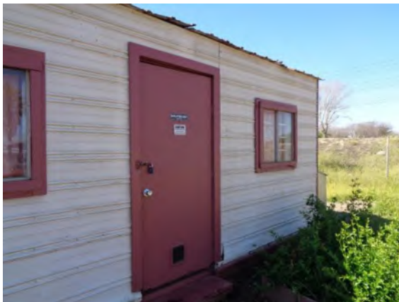
0042083a 4/2/2024 Deteriorating shed roof and old wood door rotting at bottom Barnyard Buddies
