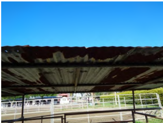
0042086a 4/2/2024 Rusting, corrugated metal roof Stalls 152-158
