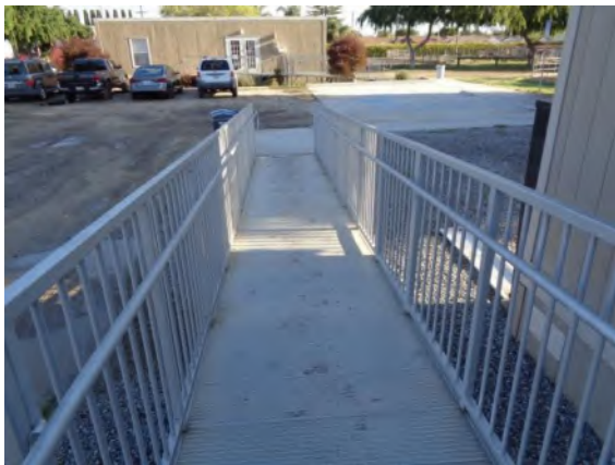
0042023a 4/2/2024 Wheelchair ramp with continuous handrails on both sides Restroom building, west elevation
