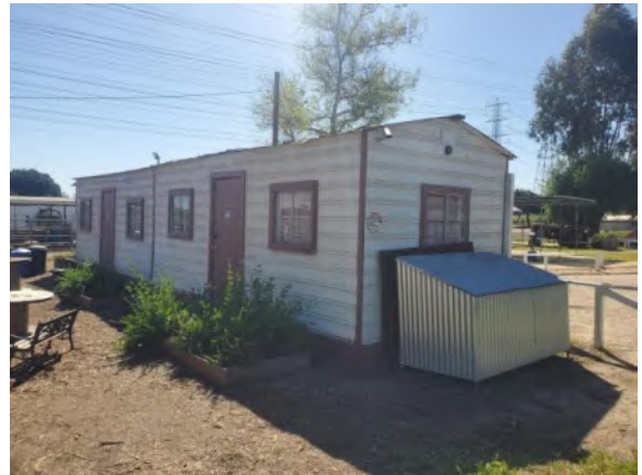
0042070e 4/2/2024 Exterior lighting Barnyard Buddies Trailer
