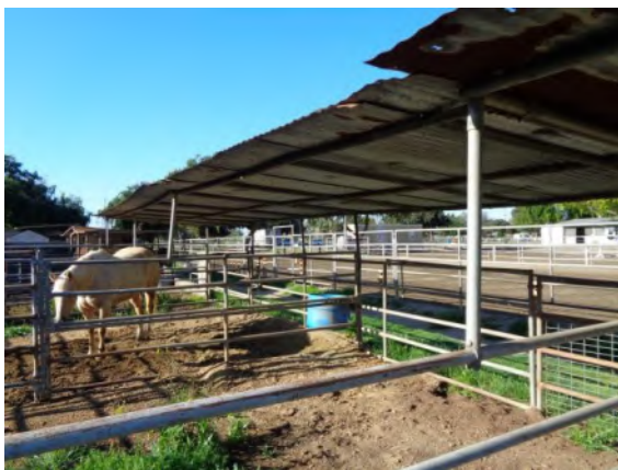
0042087a 4/2/2024 Rusting, corrugated metal roof and pipe rail fencing Stalls 152-158
