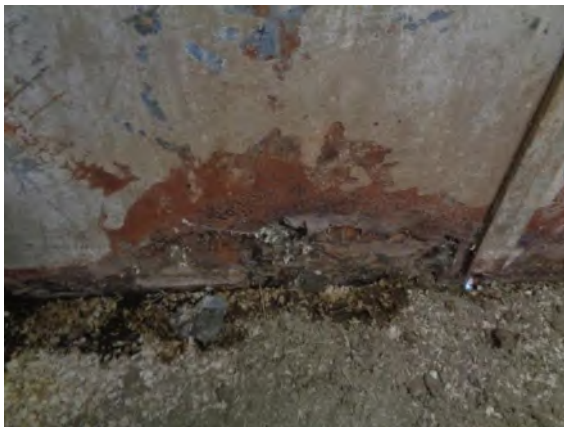
0042032a 4/2/2024 Rusting of metal clad wall panels in stall 2 Barn 1-29 interior
