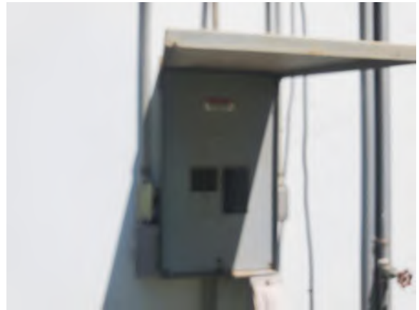
0042094e 4/2/2024 Main distribution panelboard Barn 30-39
