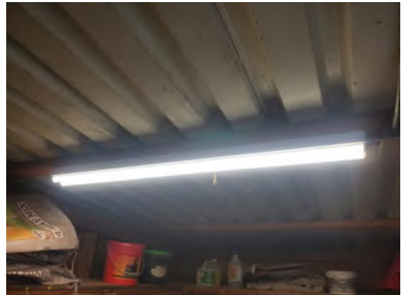
0042061e 4/2/2024 Updated interior lighting Barn 1-29, storage
