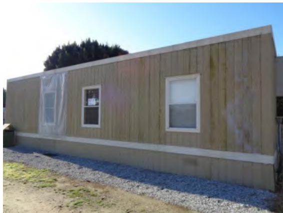
0042011a 4/2/2024 Painted T-111 plywood siding and skirting, water stains, and plastic sheeting over leaks Office, north elevation
