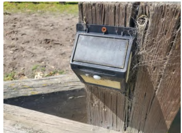
0042086e 4/2/2024 Surface-mounted, solar powered lighting Road near Dry Lots
