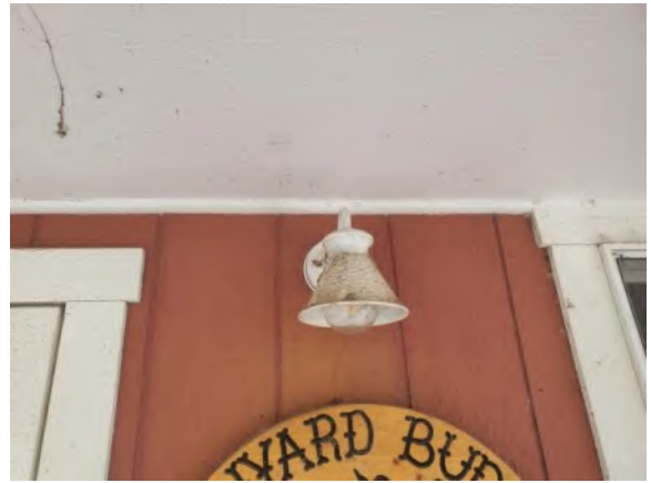
0042067e 4/2/2024 Surface-mounted decorative light fixture Barnyard Buddies Office, exterior
