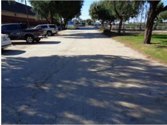
0042123a 4/2/2024 Asphalt entrance road with block cracking Roadway
