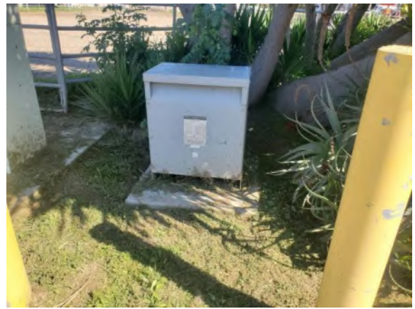
0042065e 4/2/2024 50-kVA cellular network transformer Site near Arena E
