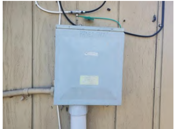
0042025e 4/2/2024 100-amp panelboard Office, exterior
