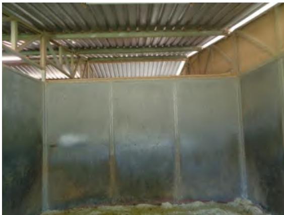
0042038a 4/2/2024 Stall 29, composite metal clad wall panels, rusting at bottom Barn 1-29 interior
