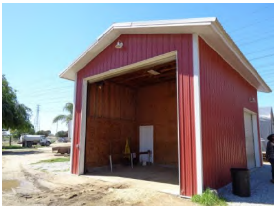
0042063a 4/2/2024 Corrugated metal exterior wall and large opening for overhead door Hay barn, east elevation
