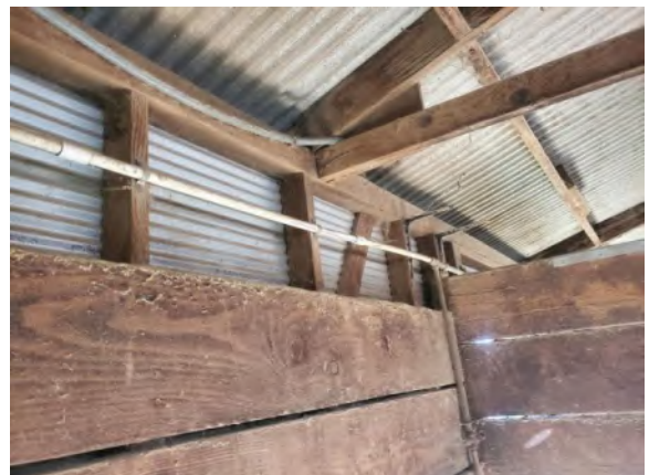
0042039e 4/2/2024 PVC water piping Stalls 170-172
