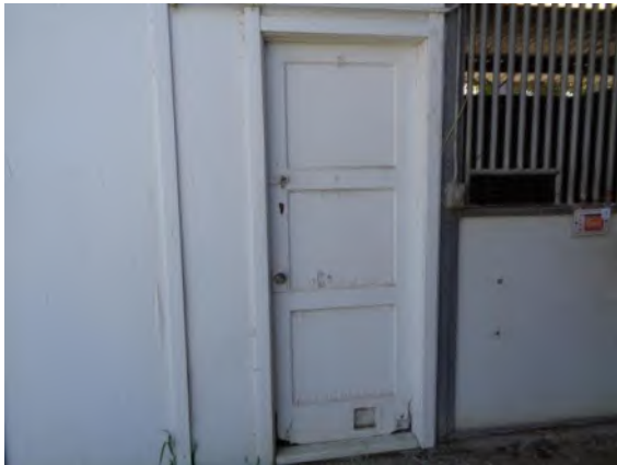
0042041a 4/2/2024 Wood door with knob hardware to storage shed Barn 1-29, north elevation
