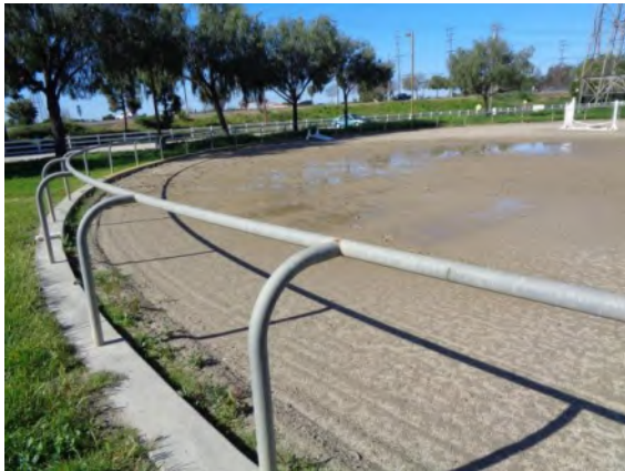
0042131a 4/2/2024 Standing water Arena A
