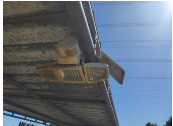
0042077e 4/2/2024 Customer-owned exterior solar powered light Stalls 63-70
