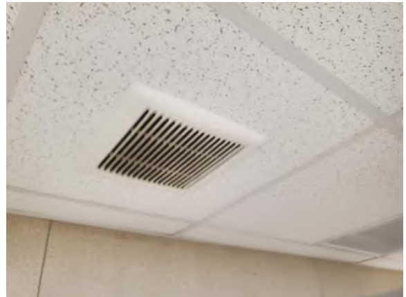
0042008e 4/2/2024 Restroom odor fan Restroom Building, men's restroom
