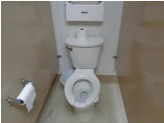
0042016a 4/2/2024 Standard toilet stall with flush-tank water closet Restroom Building, women's restroom
