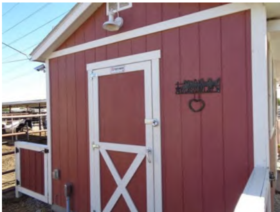
0042075a 4/2/2024 Painted wood siding and door with lever hardware Barnyard Buddies office
