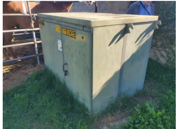
0042046e 4/2/2024 Utility-owned main power transformer Site
