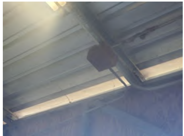
0042054e 4/2/2024 Severely corroded electrical junction box Barn 1-29
