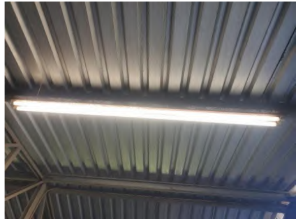
0042053e 4/2/2024 Corroded surface-mounted light fixture with T12 lamps Barn 1-29
