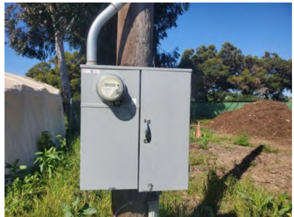
0042066e 4/2/2024 Electric meter Site near Dry Lot #4
