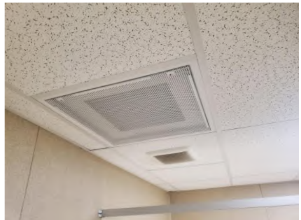
0042009e 4/2/2024 HVAC supply vent from PTAC Restroom Building, men's restroom
