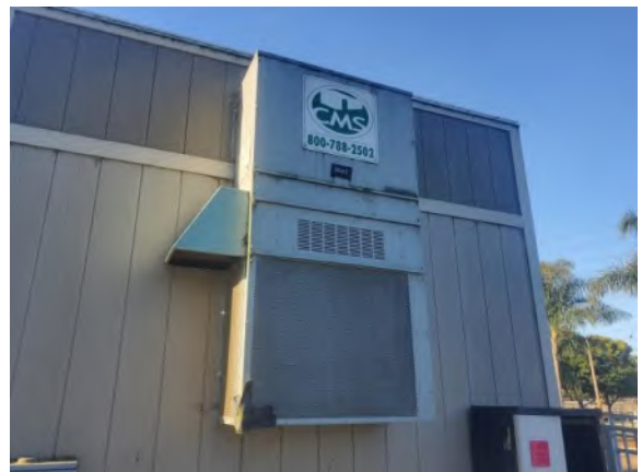
0042012e 4/2/2024 Wall-mounted package heat pump Restroom Building, exterior
