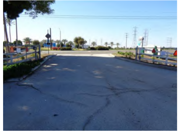
0042124a 4/2/2024 Asphalt entrance drive with block cracking Roadways
