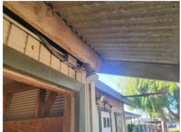
0042038e 4/2/2024 Surface-mounted flood light Stalls 170-172
