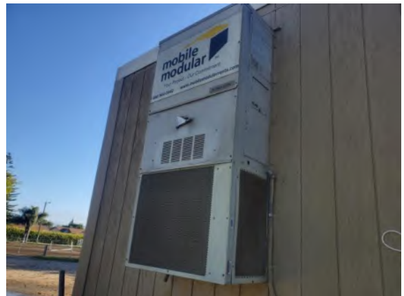
0042024e 4/2/2024 Wall-mounted package heat pump Office, exterior
