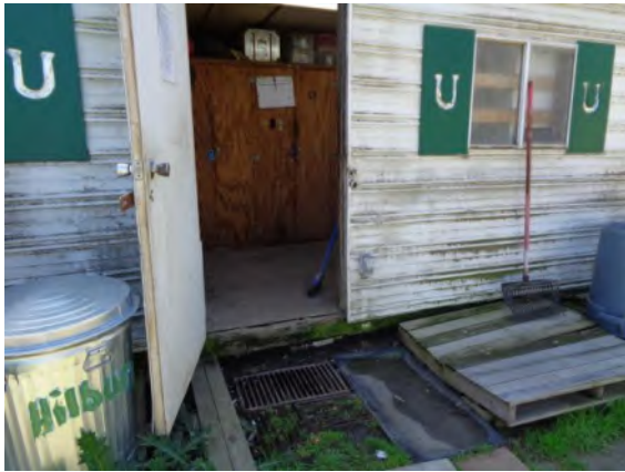
0042049a 4/2/2024 Unfinished plywood floor in shed and door with knob hardware and damage at bottom Barn 30-39, north elevation
