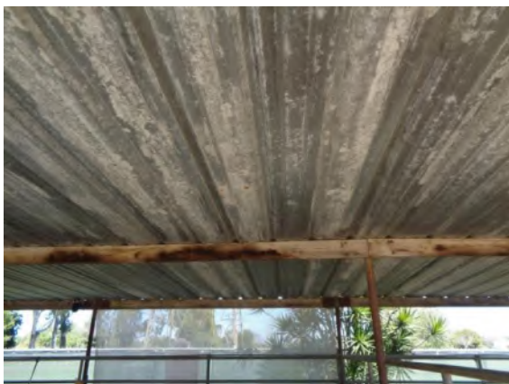
0042093a 4/2/2024 Corrugated metal roofing supported on wood stringers and pipe columns Stalls 147-151
