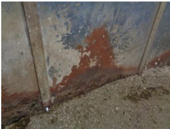
0042033a 4/2/2024 Rusting of metal clad wall panels in stall 2 Barn 1-29 interior
