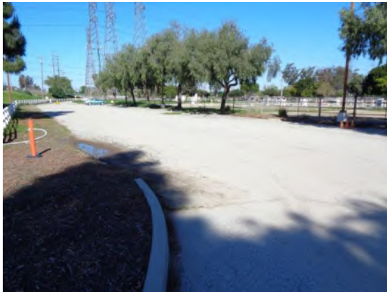
0042125a 4/2/2024 Asphalt pavement with block cracking and standing water at edge Roadways
