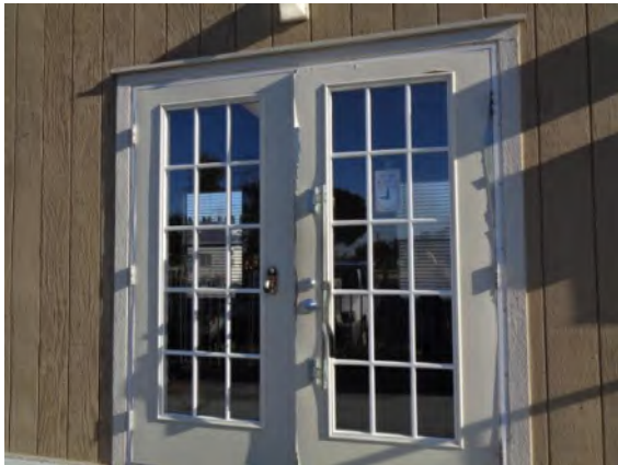
0042008a 4/2/2024 Entrance doors with glass lites, lever hardware, and peeling paint Office, south elevation
