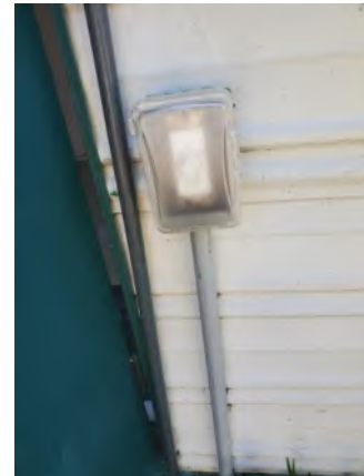
0042083e 4/2/2024 Timed electrical switch Dressage
