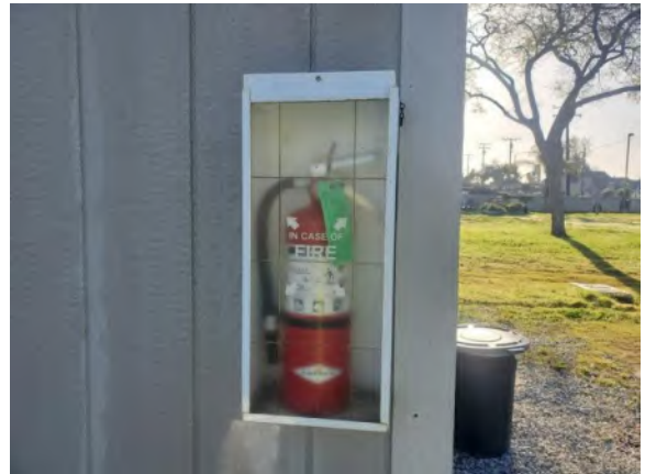
0042002e 4/2/2024 Fire extinguisher Restroom Building, exterior
