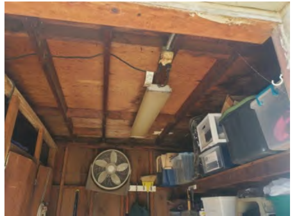
0042079e 4/2/2024 Surface mounted lighting with T12 lamps Wood Tack Shed 7-8
