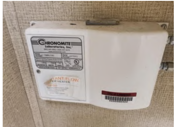
0042005e 4/2/2024 Instantaneous water heater Restroom Building, men's restroom
