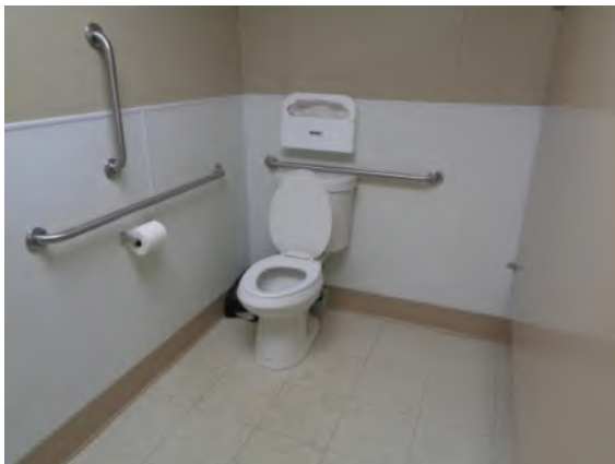
0042017a 4/2/2024 Accessible stall with flush-tank water closet and grab bars Restroom Building, women's restroom
