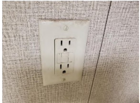
0042007e 4/2/2024 GFCI electrical outlet Restroom Building, men's restroom
