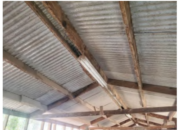
0042035e 4/2/2024 Surface-mounted lighting with T12 lamps Stalls 170-172
