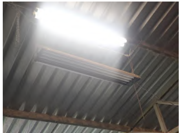
0042057e 4/2/2024 Occupant-owned infrared heater Barn 1-29
