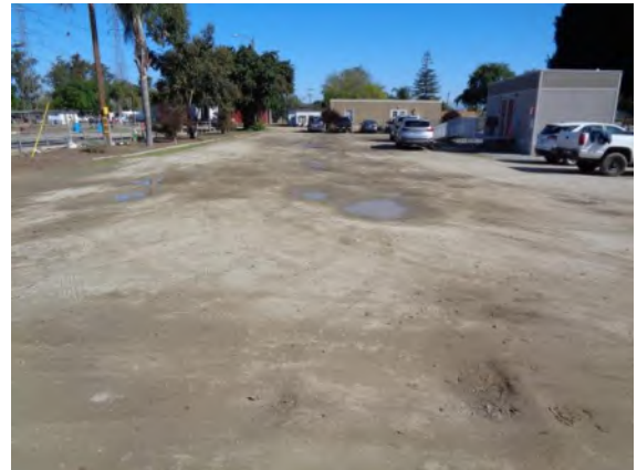
0042126a 4/2/2024 Dirt covered pavement and potholes Center roadway and parking area
