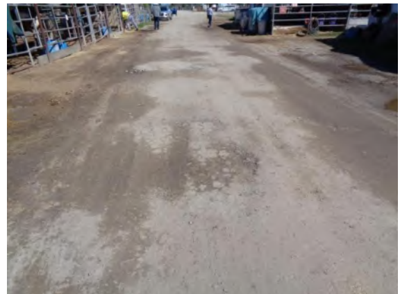
0042128a 4/2/2024 Dirt covered roadway with alligator cracking Roadway
