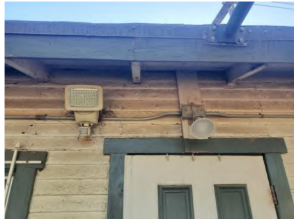
0042040e 4/2/2024 Surface-mounted light fixtures Tack Shed, exterior
